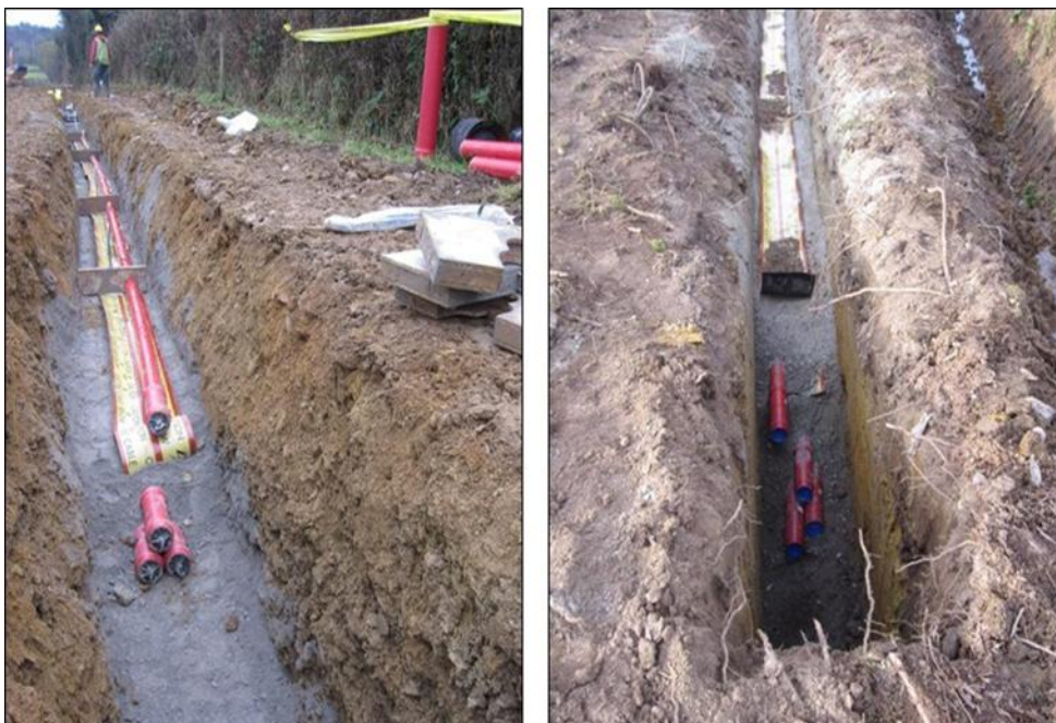
Plate 2-2 Typical Trefoil Cable Trench View
